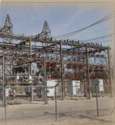
Electric substations like this one in Winchester, KY are common sights, indicative of our state's need for power for residential and industrial uses.
