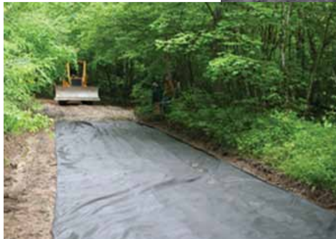
Once you have smoothed the road surface roll out the geotextile fabric (above) and dump a large load of gravel on one end. Do not drive directly on the fabric as it is subject to tearing and shifting.
