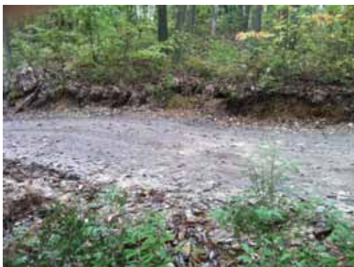
Broad based dips are a water control structure that collects water from the uphill side of the road (surface and ditches) and diverts it across the road to a stable outlet. They work best on roads with slopes of less than 10%.
