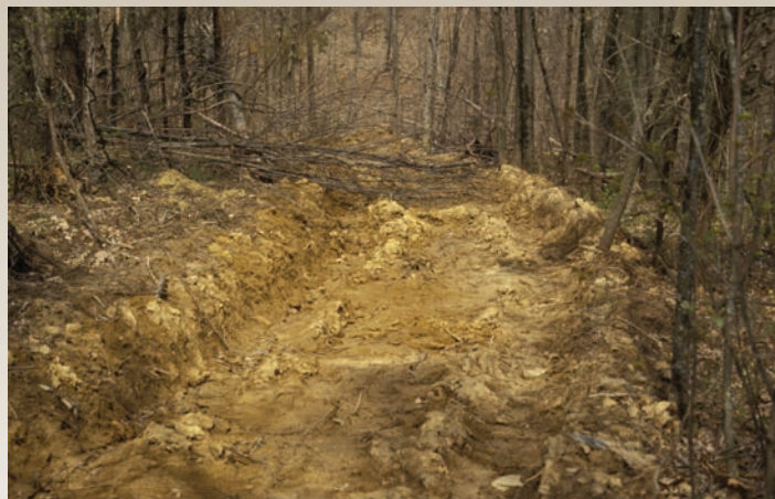
Figure 2. Under the new BMP requirements ruts like this may or may not be required to be fixed depending on whether or not they are causing a water quality problem or not.
